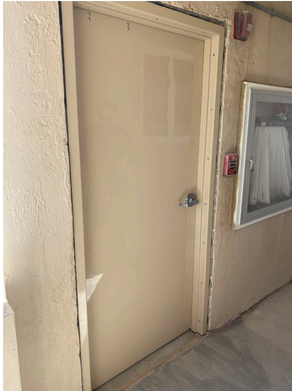
Picture 7: Typical fastening of stairwell doors
